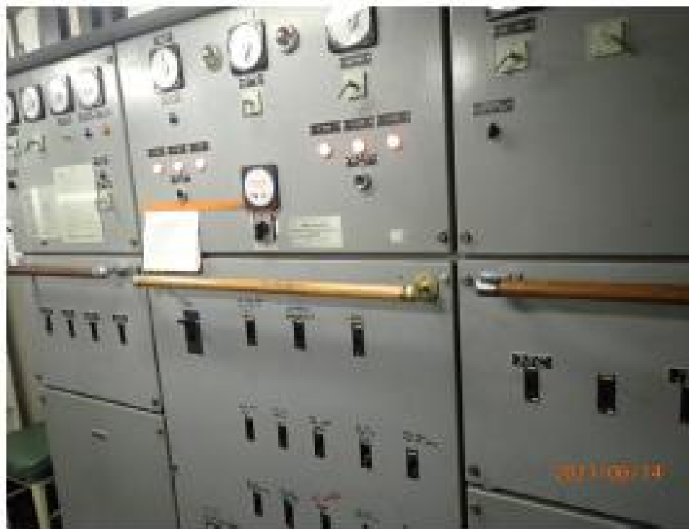
MAIN ELECTRICAL PANEL
